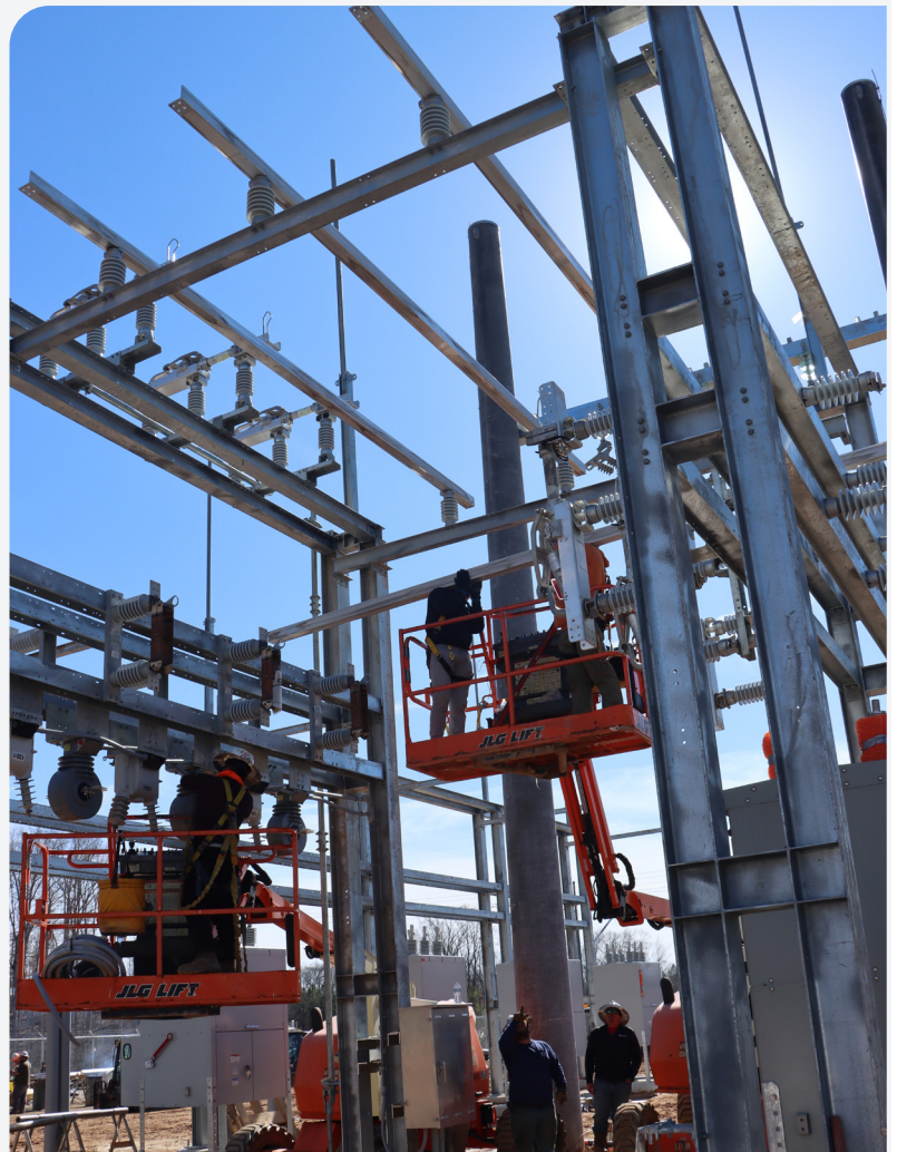
Photo courtesy of Georgia Transmission Corporation
